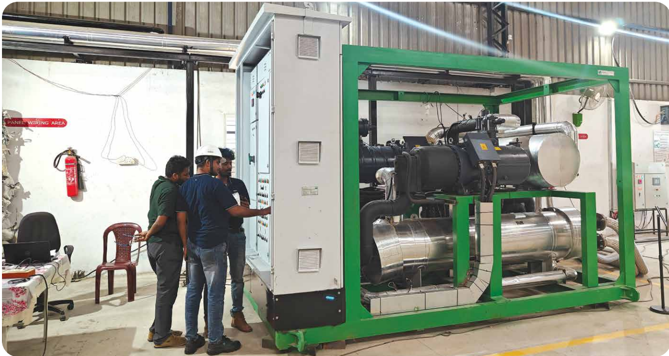
High-temperature steam generating heat pump (site and technology courtesy: TRIGeN Decarbonisation)
